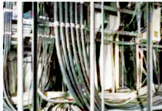
Cable distribution is complicated with high fire load
